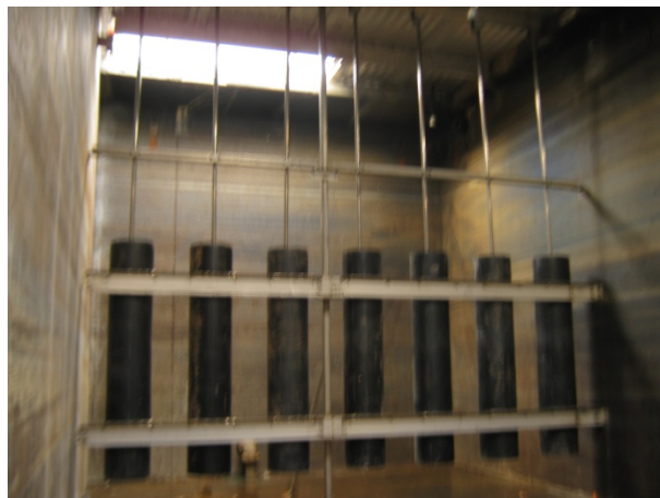
Shear Tube Aeration Equipment Under the AirBeam™ Cover
