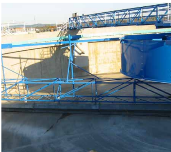
Scum box skimming system
