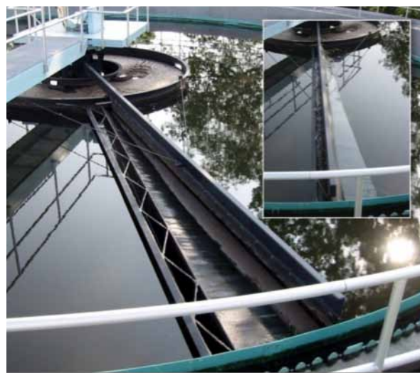
Full trough skimmer (FTS) system
