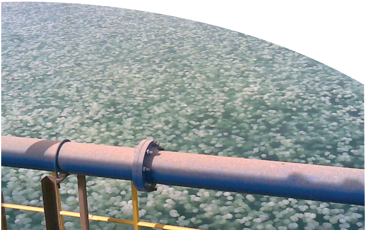
Large influx of jelly fish at a power plant cooling water intake
