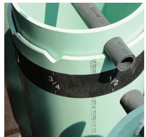
CLEARLY MARKED VALVE POSITION
