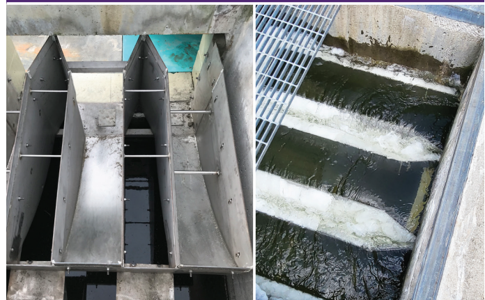
SERPENTINE WEIR CONTROLS
