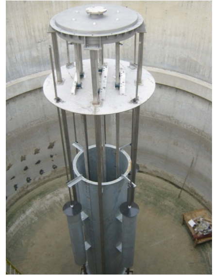
MEDT Aeration Equipment Under the Airbeam™ Cover
