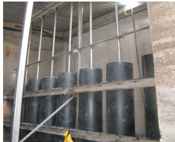
Shear Tube Aeration Equipment Under the AirBeam™ Cover
