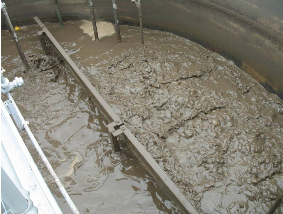
Woodside Membrane Thickening and Sludge Holding Tank
