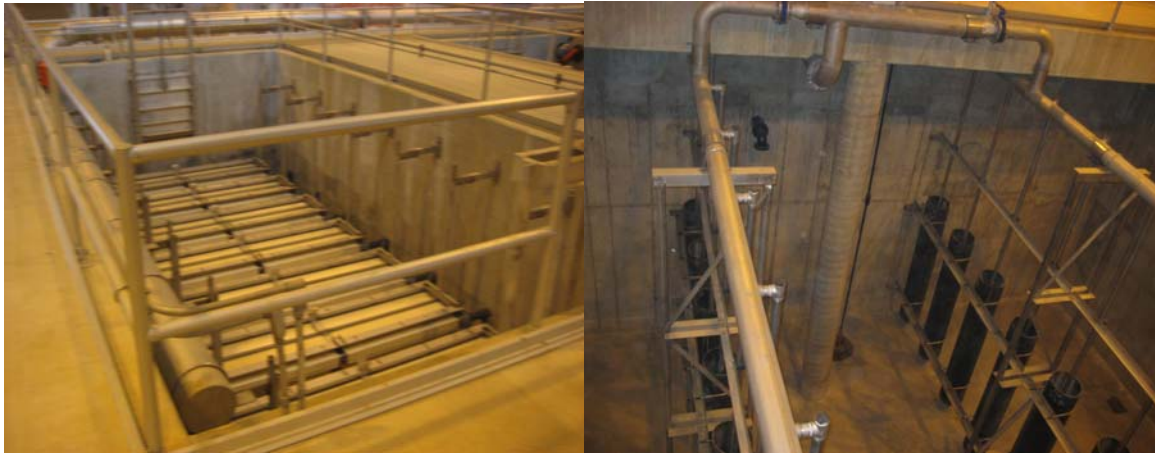
Figure 5. Union Rome WWTP Membrane Thickening Aerobic Digestion System (Membrane Thickening Tank shown on the left, Aerobic Digester shown on the right)
